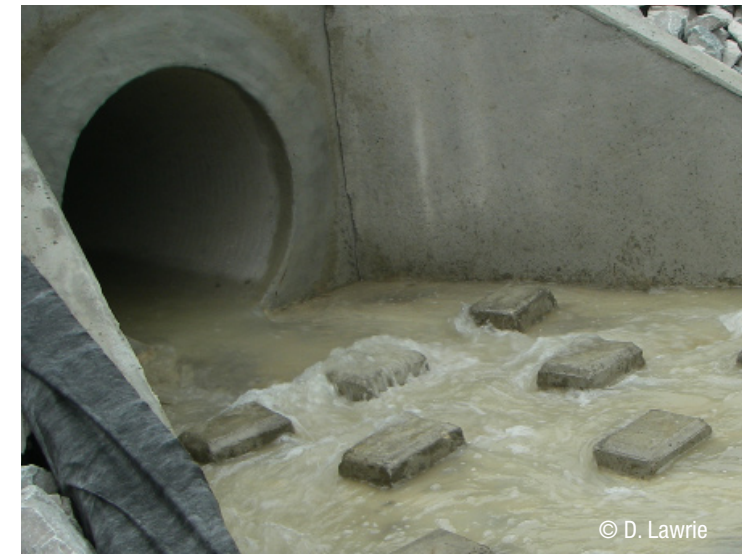
© D. Lawrie Stormwater discharge from construction site
